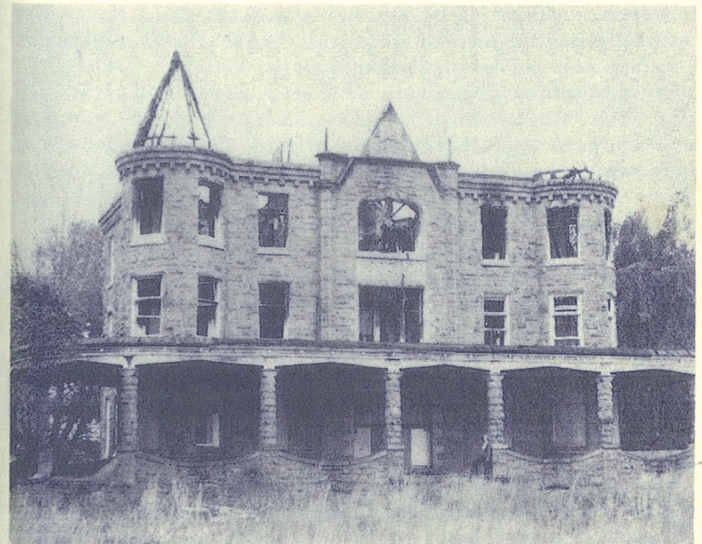
The Bergdoll Broomall castle, built in 1907. Courtesy of the Philadelphia Bulletin. The Broomall castle now lies in ruins after what police term a "suspicious" fire on March 24, 1976. Photo by Ronald Dell.
